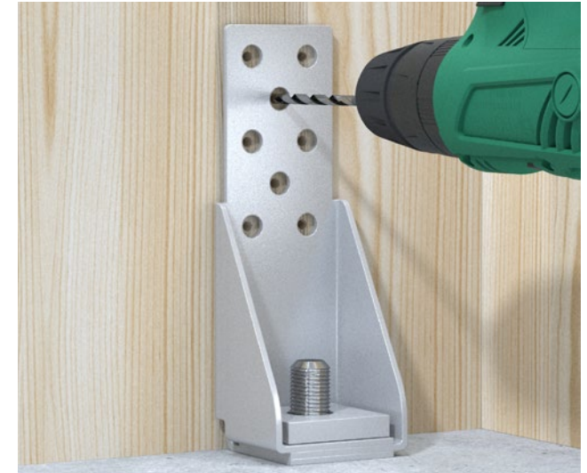
Figure 2 Installation of the Multinail tie-down bracket with washer. Pre-drill for all screws using a 5.0mm diameter drill bit
